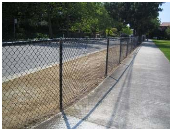
Degraded chain link fence
