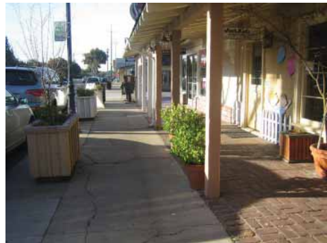
Existing sidewalk paving is cracked and inconsistent in color.
