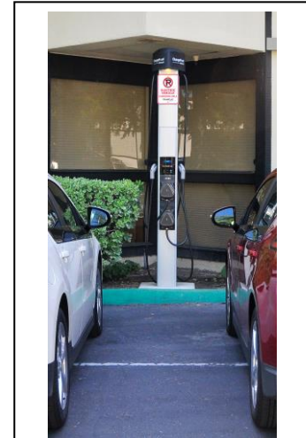
Figure 2-8 ChargePoint America Charging Station
