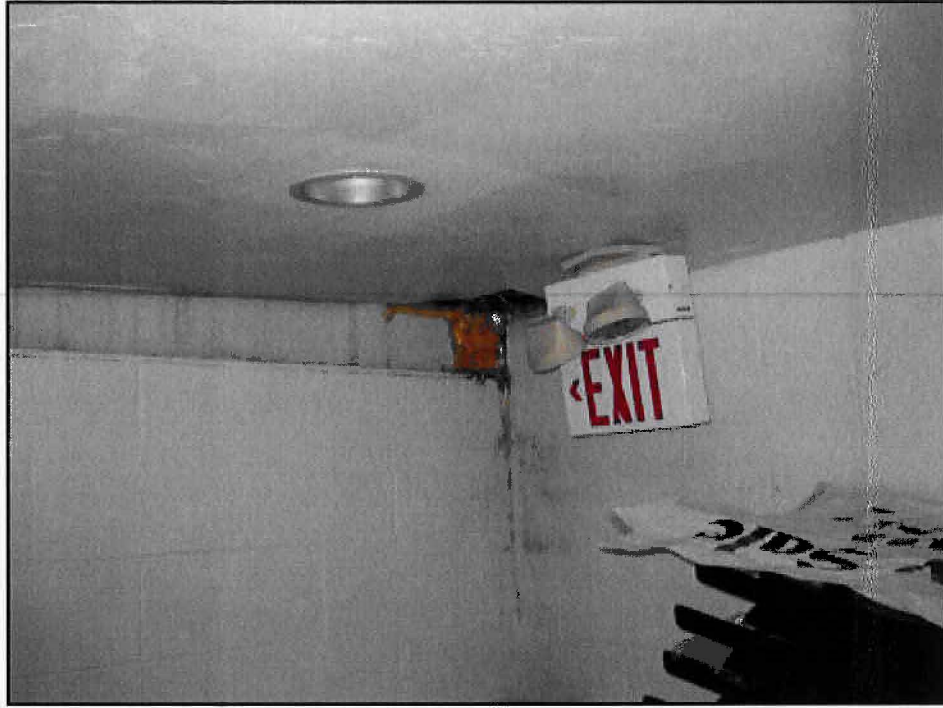
E09-581; Mold/water intrusion at basement area.
