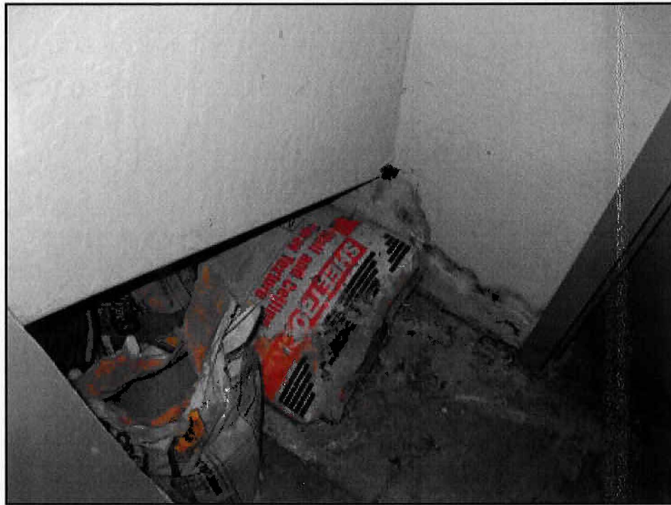
E09-581; Mold/water intrusion at basement area.
