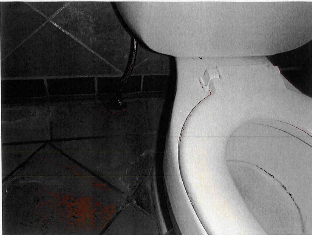
Notice Water Staining on floor area
