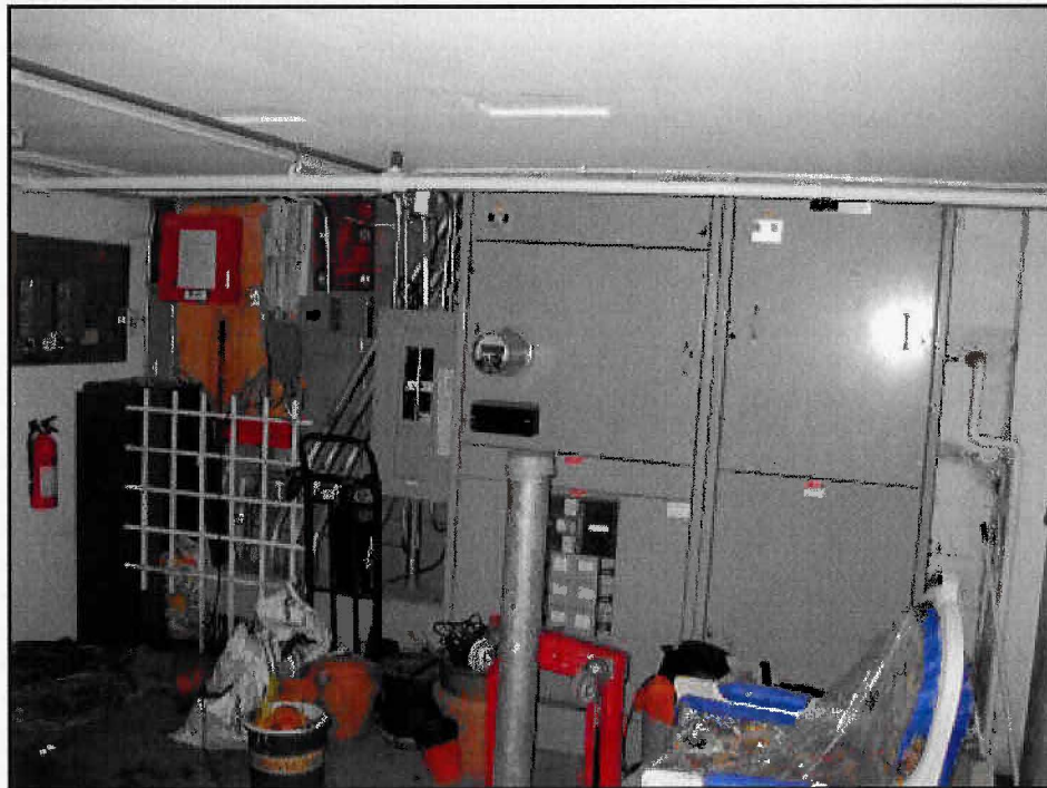
E09-581; electrical service
