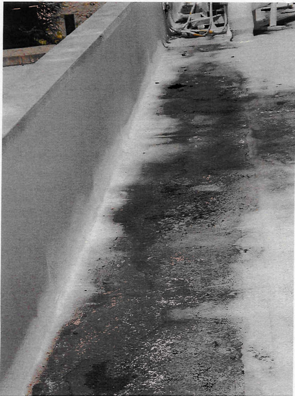
Roof Area with visible evidence of water stagnation
