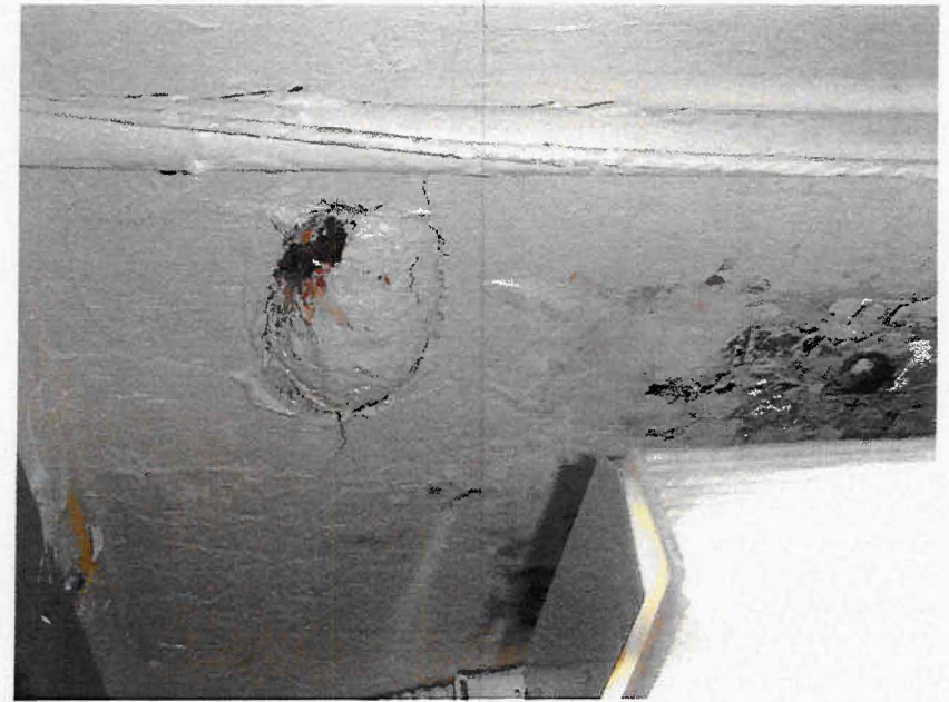
Staining/discoloration on ceiling area
