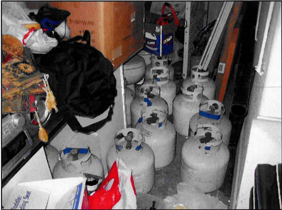
E09-581; propane tank storage
