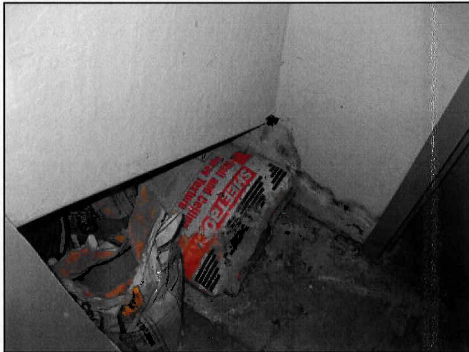
E09-581; Mold/water intrusion at basement area.
