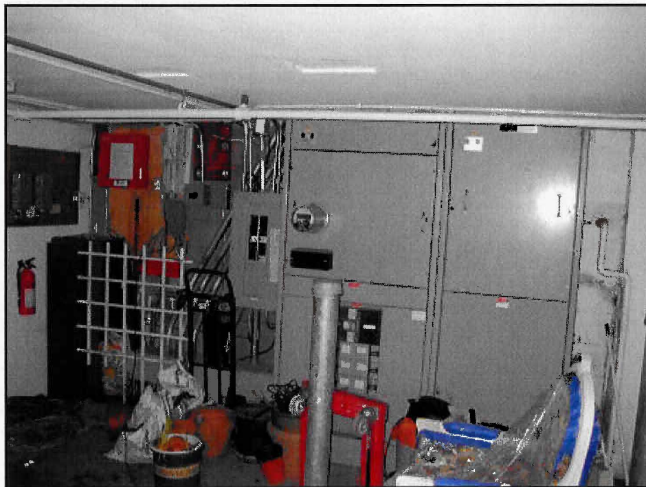
E09-581; electrical service
