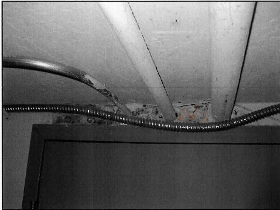
E09-581; Mold/water intrusion at basement/storage area
