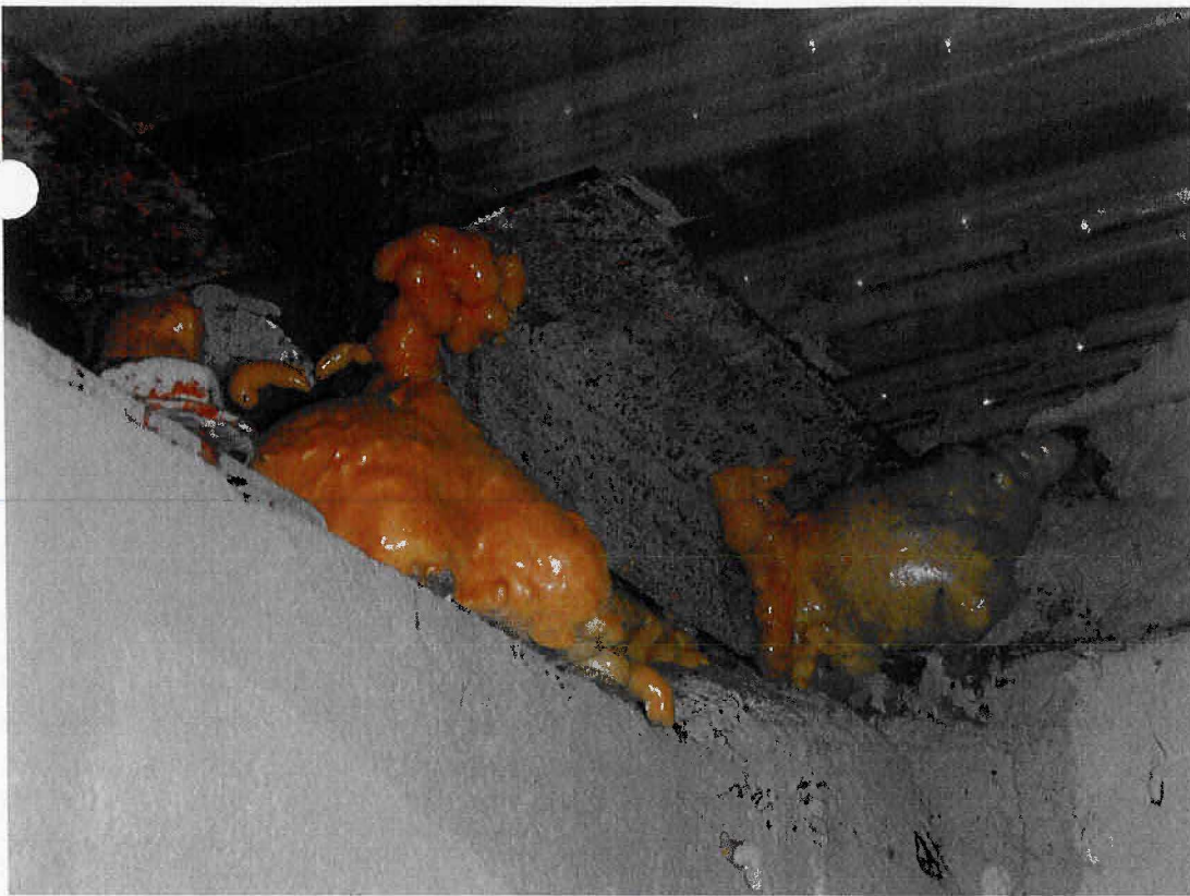
Visible evidence of water intrusion at top portion of walls
