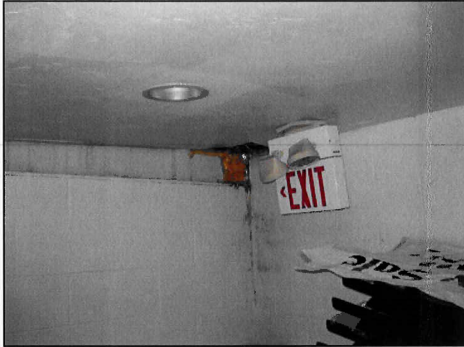
E09-581; Mold/water intrusion at basement area.
