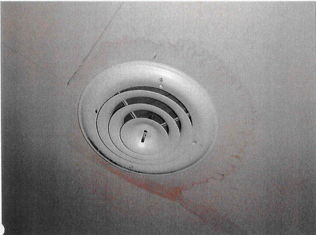
Notice Water Staining around Ceiling Vent 2nd Level - Wine Storage Area
